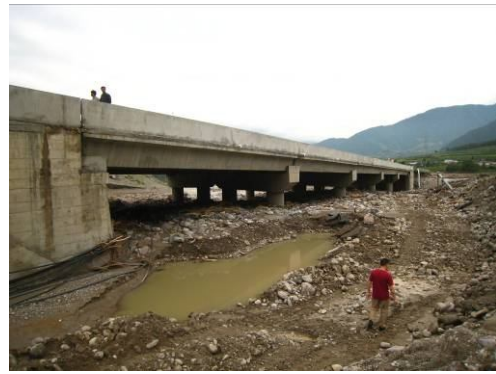
图 7 墩台受冲击破坏但桥面通行仍可维持 Fig.7 Traffic function of bridge fairly maintained with piers being impacted by debris flow
