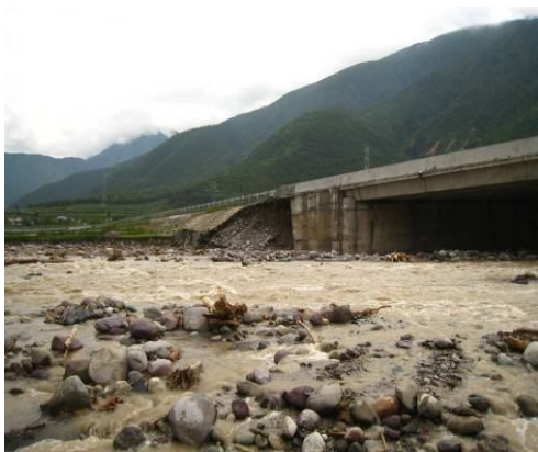
图 6 安宁河桥受泥石流冲刷致淤堵 Fig.6 Anninghe bridge impacted and blocked by debris flow
